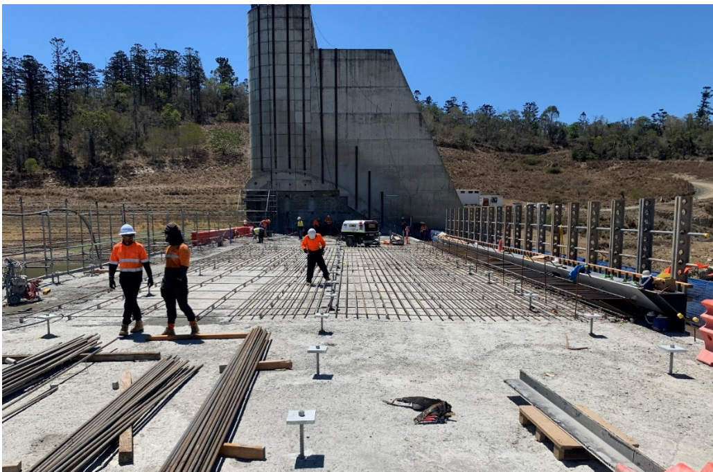
Figure 1: Steel reinforcement in preparation for concrete pours to construct the new crest
