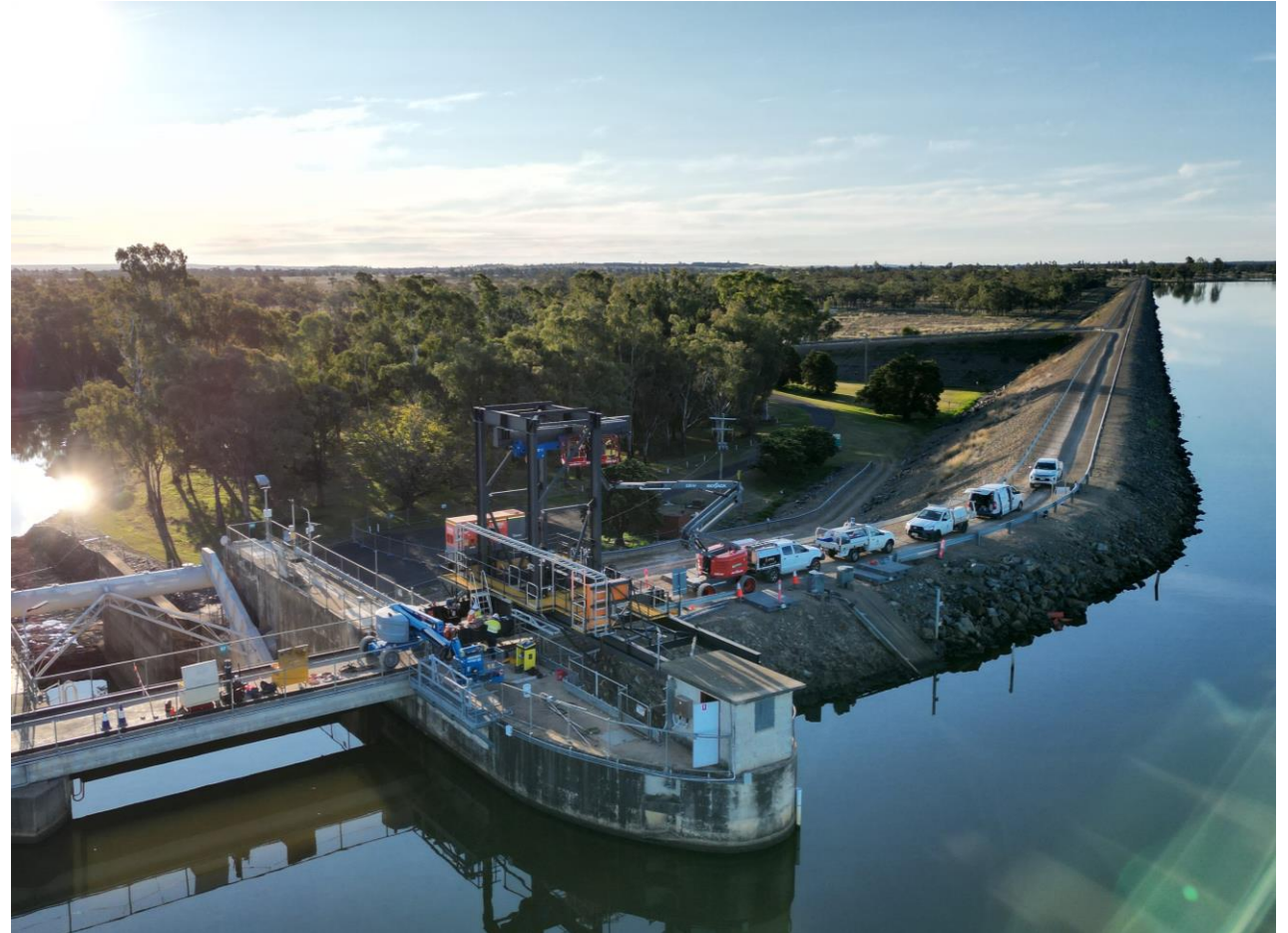
Example of works on a spillway - Sunwater's Coolmunda Dam Variable Counterweight Works
